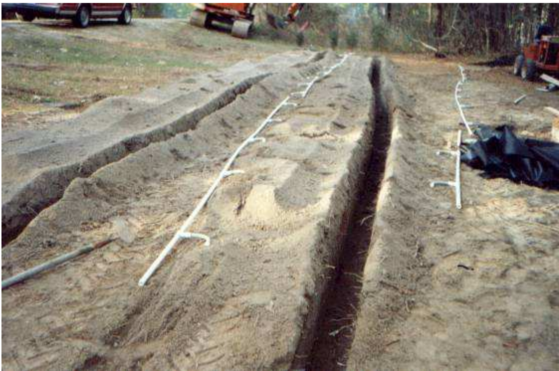
Figure 4. Examples of underground emitters placed in a 10" trench and filled with chopped rubber and covered with 100 mesh groundcloth
