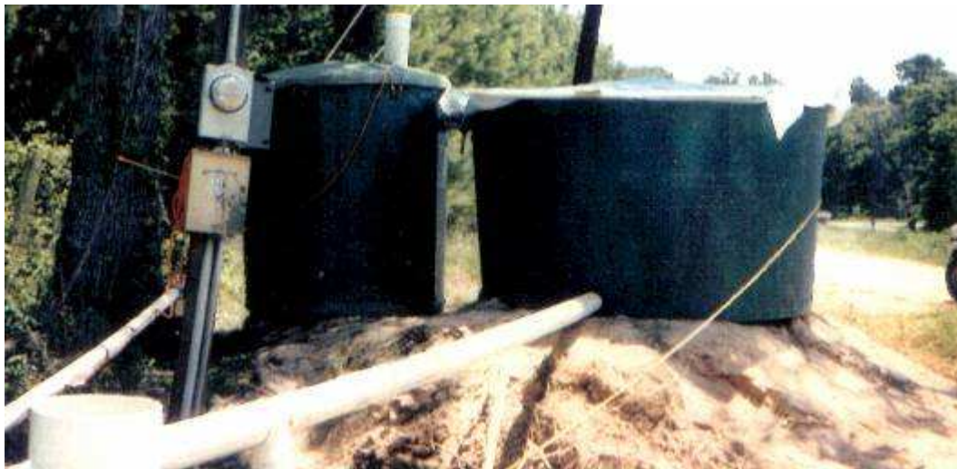
Figure 1. Tank test system using vacuum microbubble aeration pretreatment at Texas Landing on Lake Livingston.
