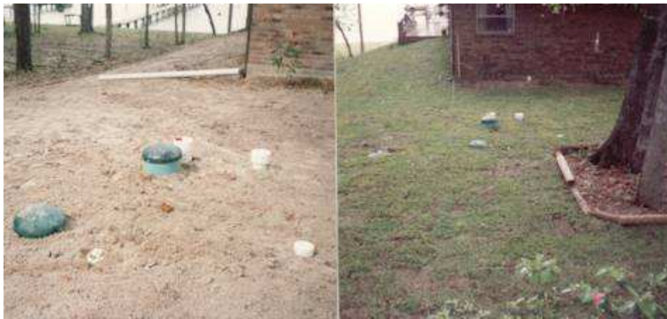
Figure 5. Corrective applications to the existing tank system of the Cartier site.
