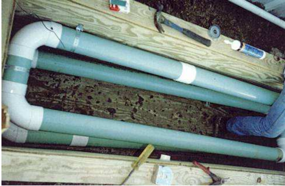
Figure 5. Cooling chamber added to cool kitchen wastewater prior to entering the #1 1250-gallon trash tank.
