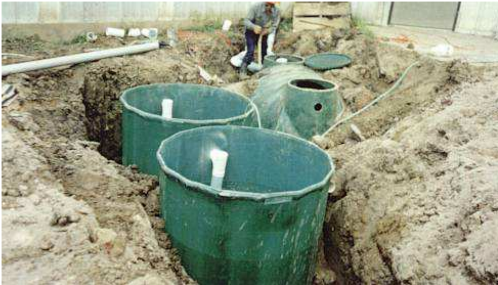
Figure 2. Blackwater and mixer tanks pretreatment for the Hydro-Flo aerator units.
