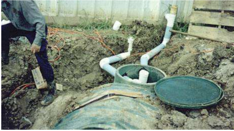
Figure 1. Initial excavation and emplacement of a 1250-gallon digesting tank at LoneStar Charlie's.
