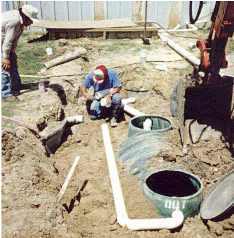
Figure 6. Addition of second 1250-gallon trash tank pretreatment for Hydro-Flo aeration units.
